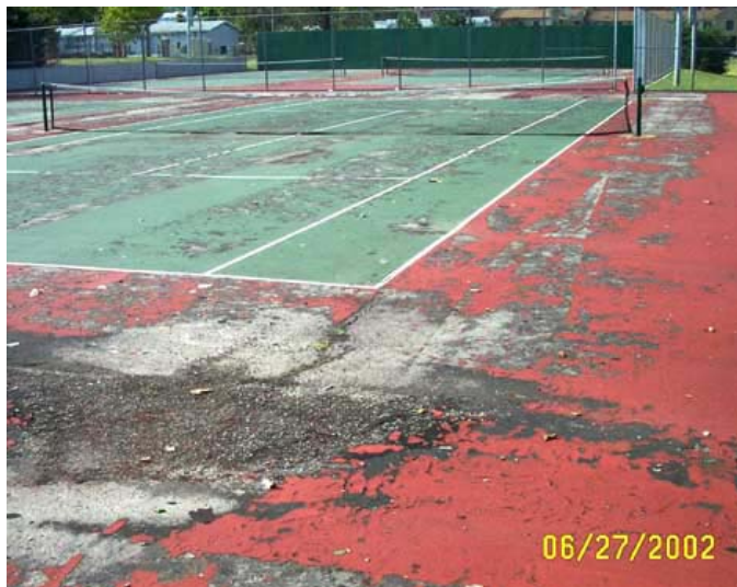
Crumbling tennis court surface – The Parade, 6/27/02
