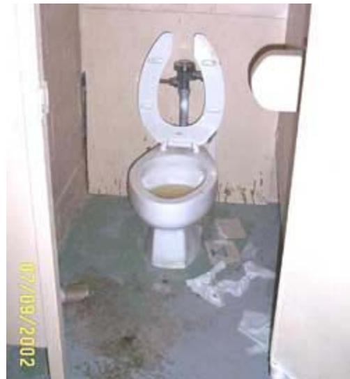
Dirty restroom floor littered with paper - Loose Park, 7/9/02
