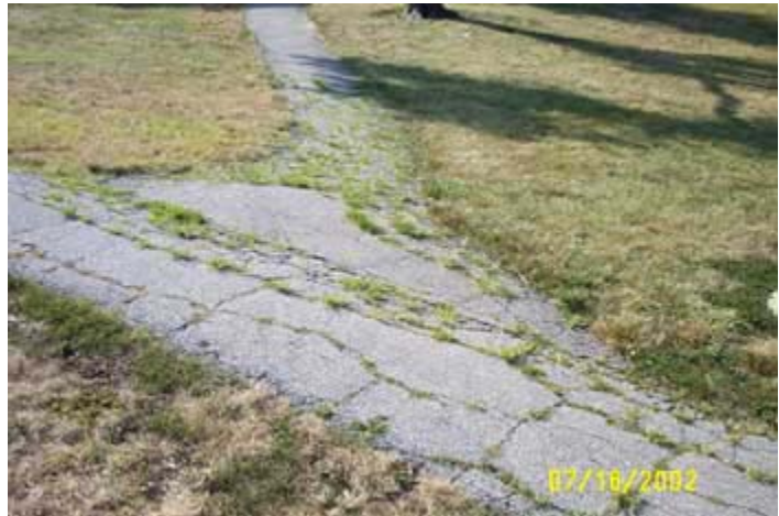
Deteriorating asphalt path - Westwood Park, 7/18/02
