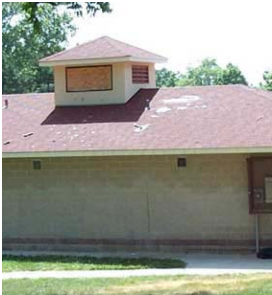
Peeling roof tiles and boarded up opening at pool building – Budd Park, 7/1/02
