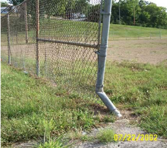
Damaged backstop post - Liberty Park, 7/22/02
