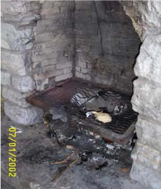
Rusted grill at shelter - Budd Park, 7/1/02
