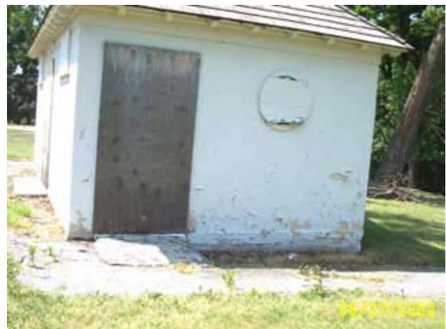
Peeling paint on boarded up outbuilding - Crews Square, 6/27/02
