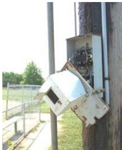
Cover hanging off breaker box - Observation Park, 7/9/02
