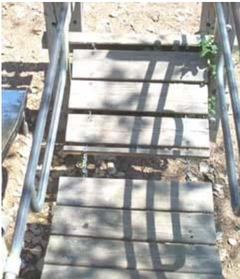
Playground bridge with missing board - Noble Park, 7/18/02
