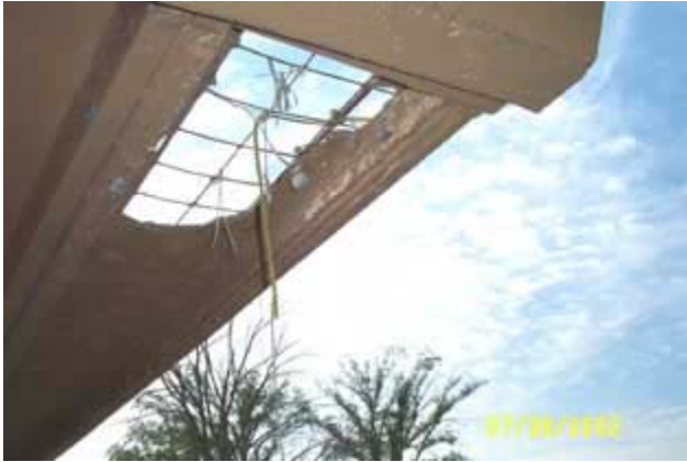
Hole in shelter roof - Englewood Park, 7/26/02
