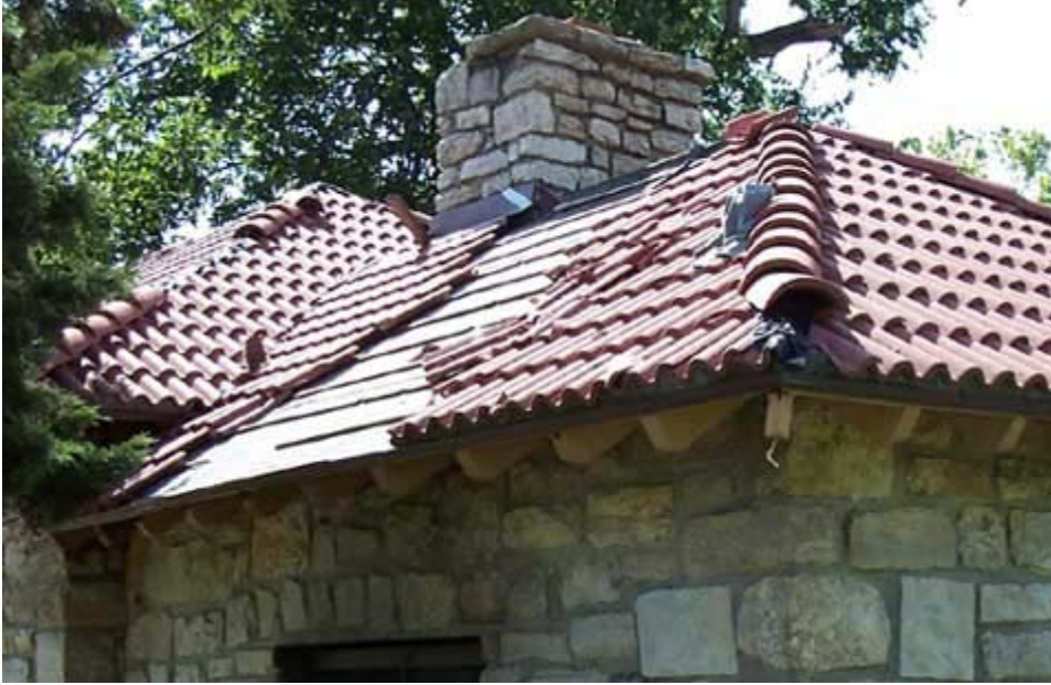
Missing clay roof tiles on stone shelter - Budd Park, 7/1/02
