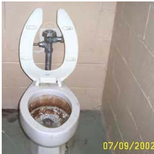
Stained toilet bowl - Loose Park, 7/9/02
