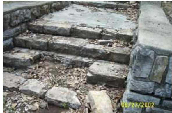
Crumbling and debris covered stone steps - Crews Square, 6/27/02
