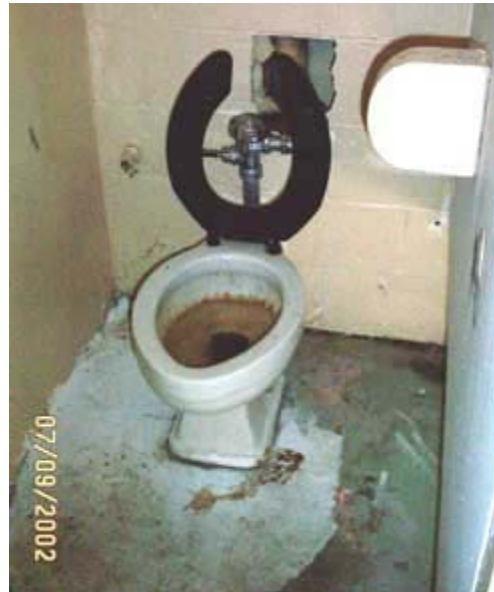
Unsanitary toilet and floor in men's restroom - Loose Park, 7/9/02
