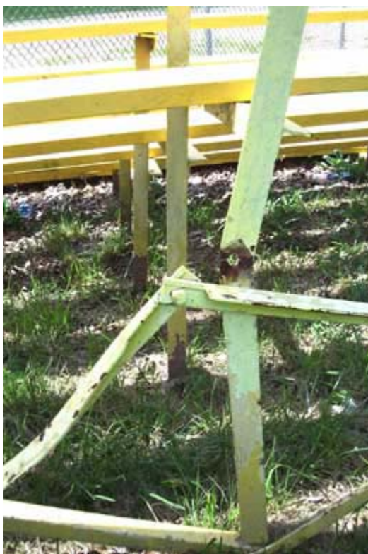
Broken support member on back of bleachers - Crestview Park, 6/12/02
