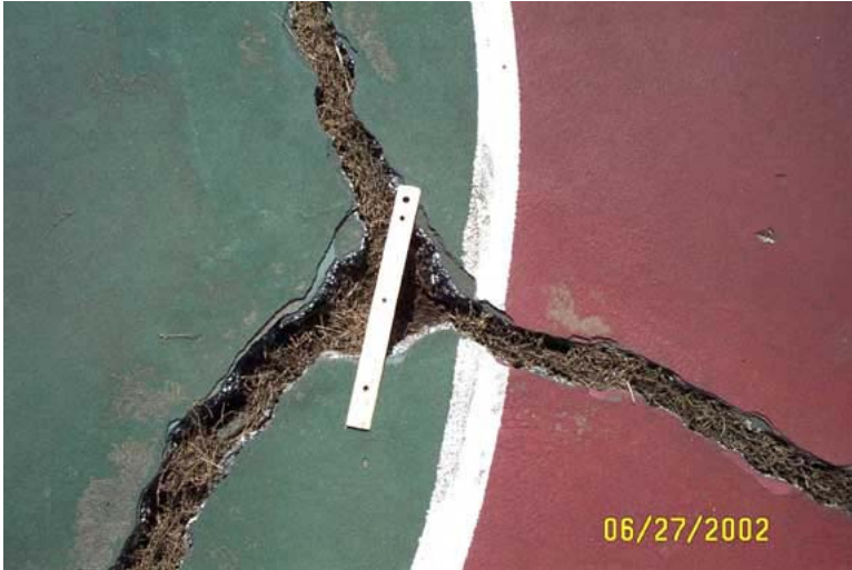
Ruler measuring 6" crack on basketball court - Crews Square, 6/27/02
