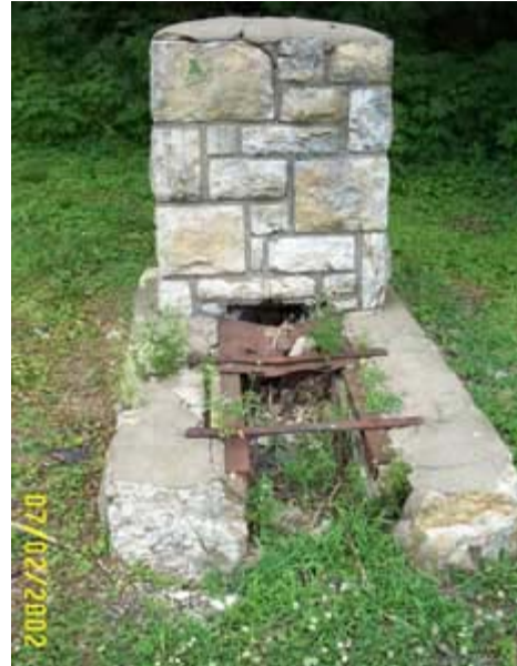
Damaged and rusted grill with weeds growing out of it - Blenheim Park, 7/2/02
