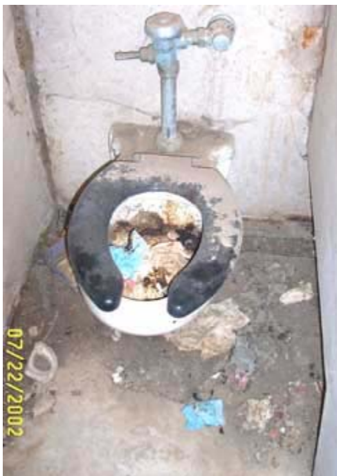
Clogged toilet, with littered and dirty restroom floor - Liberty Park, 7/22/02
