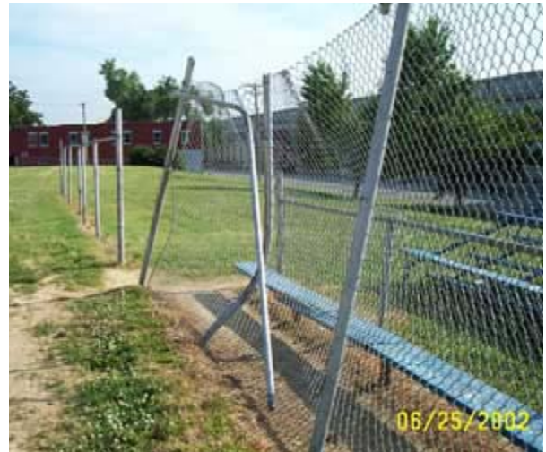
Partially collapsed backstop - Sheffield Park, 6/25/02
