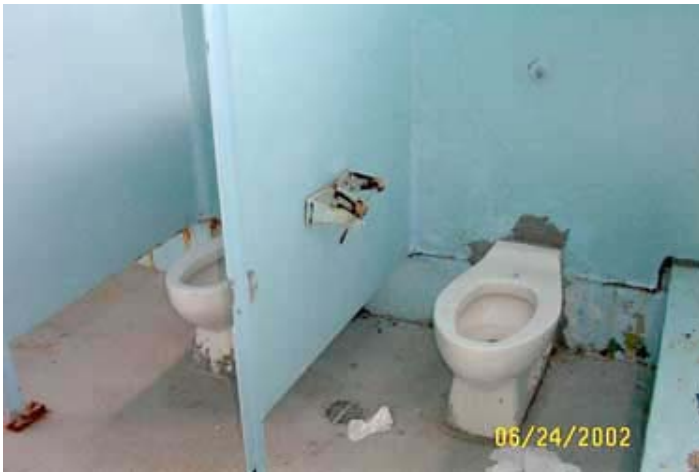
Men's restroom with rusted walls and peeling paint – Sunnyside Park, 6/24/02
